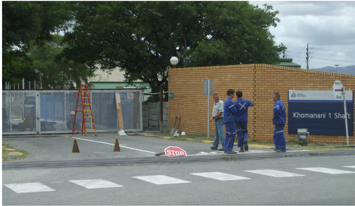
Amplats getting additional gates welded onto the entrance of its Khomanani 1 Shaft in Rustenburg as workers laid down tools in protest against the threatened closure.
